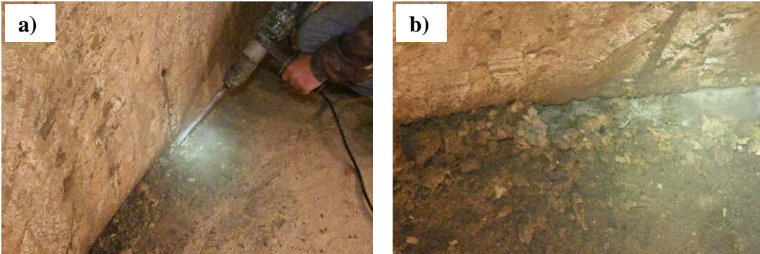
Figure 31. Groove for floor joint chipped out using chipping hammer to create a groove approximately 1 inch in depth.
