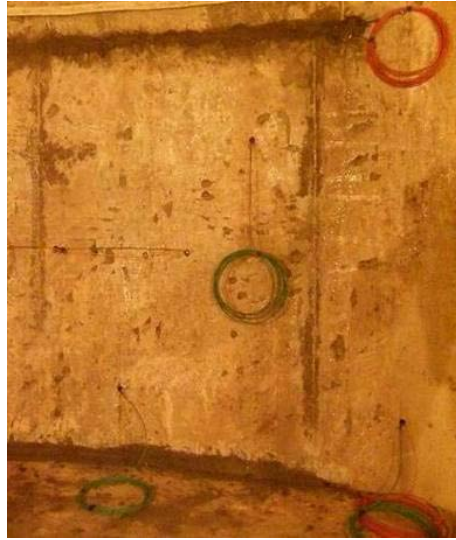
Figure 37. Locations of cathodes (green cables) in relation to each other and to anodes (red cables).
