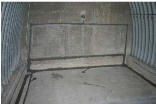
Finished EOP system installation
