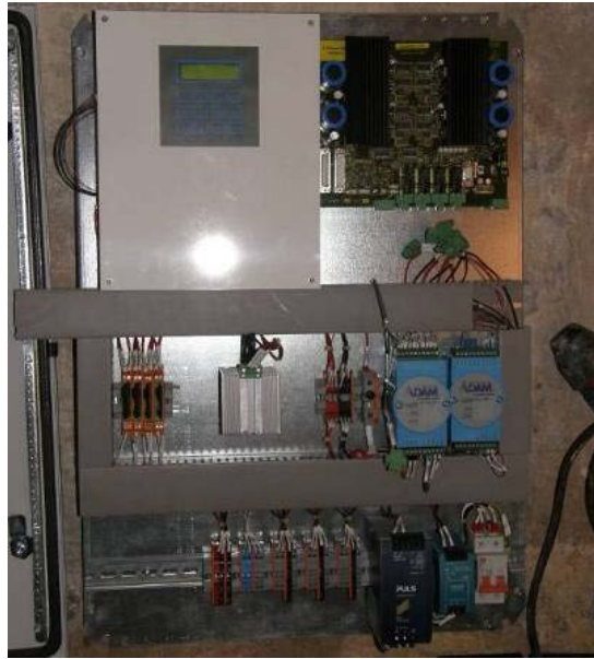
Figure 26. DC voltage controlled pulse unit installed at Trinity Dam for the EOP system.
