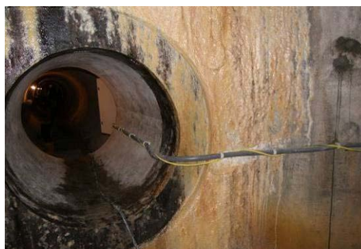
Figure 44. The conduit containing the anode header cable, cathode header cable, and rebar cable. The unit is powered by the yellow extension cord wrapped around the conduit.
