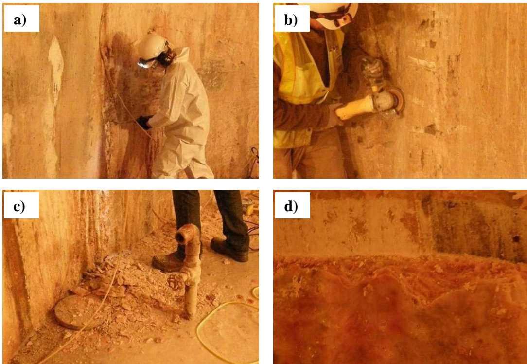
Figure 27. Removal of calcite from the concrete wall in the bonnet chamber using a chipping hammer (a) and grinder (b). The volume of calcite removed is shown in (c). Deposits on the wall were an average of 0.5 to 1 inch thick (d).
