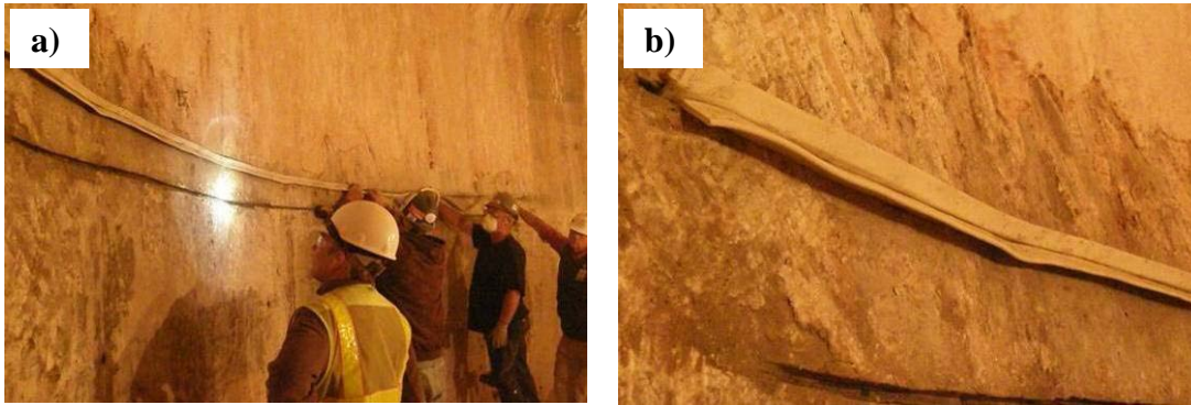
Figure 29. Installation of weather strip to act as a drip tray for water dripping down from above.
