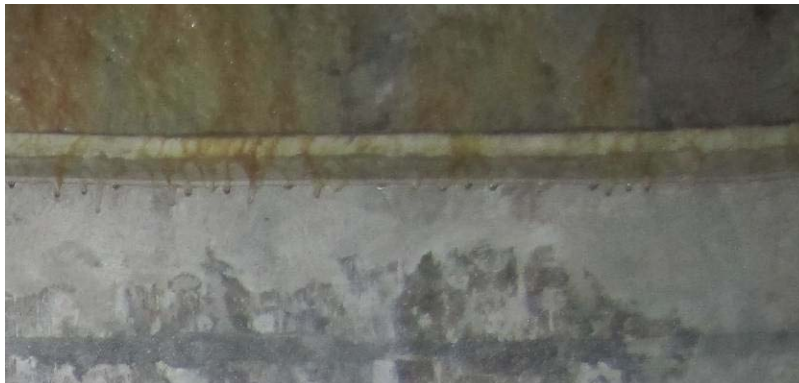
Figure 53. Visible water overflowing the drip tray, allowing water to fall onto the wall and junction boxes below. Note the color of the streaks of water, indicating that the water is rich in calcium carbonate.
