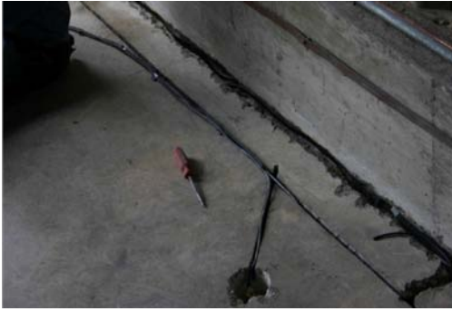
Cable runs and grooves
