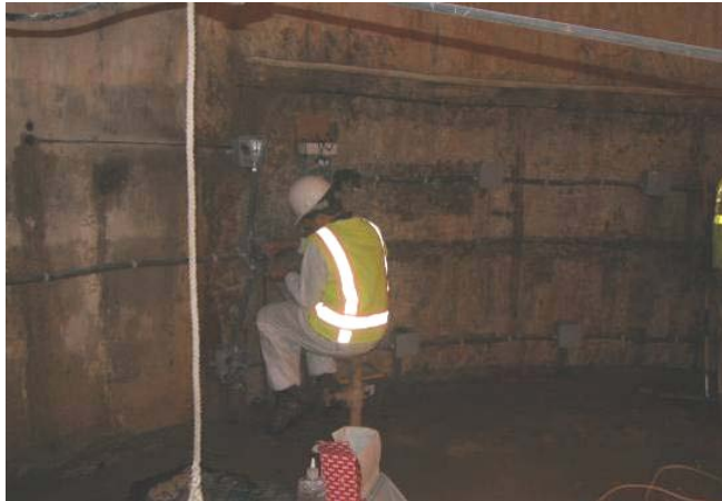
Figure 41. All cables were terminated in a main junction box. The cathode cables were connected to a main cathode header cable, all the anode cables were connected to a main anode header cable, and the main header cables and a cable connected to the rebar were run through conduit to the system controller.
